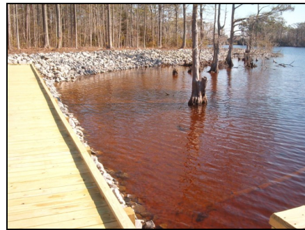
The public shoreline has been stabilized and protected with 160 feet of bulkhead and 325 feet of rock rip rap.
